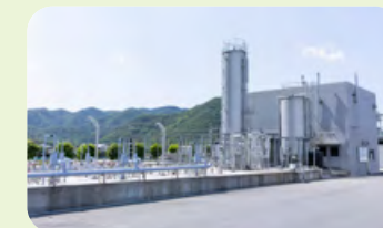
Wastewater treatment facility
