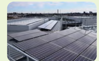
Solar panels at the Yakult Central Institute
