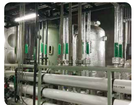
Water treatment facility
