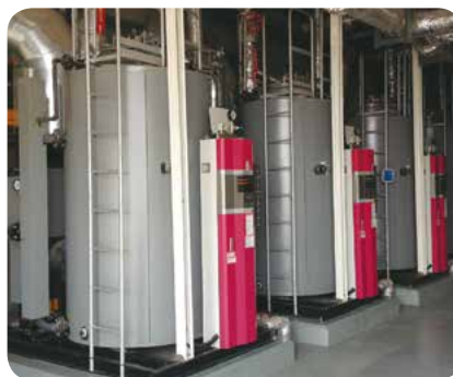
Natural gas boiler
