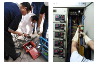
Electrical safety self-inspection at the Shanghai Plant
