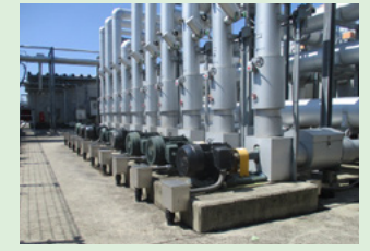
Cooling water pump, Fukushima Plant
